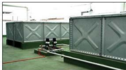
Picture 1.9: Rain Water Harvest Water Tank Source: KETTHA building
