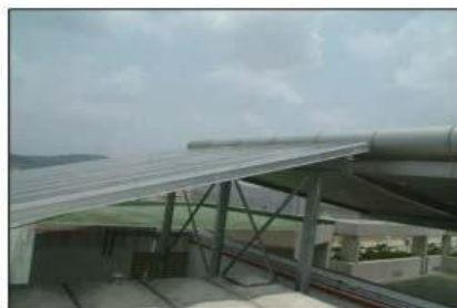
Picture 1.8: Solar Photovoltaic System at the Roof Source: KETTHA building
