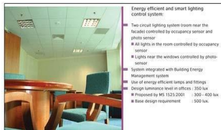
Picture 1.5: Lighting Control System Source: KETTHA building
