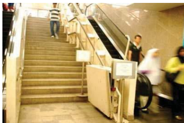
Figure8: Platform Lift Installed at the Staircase Leading from Kuala Lumpur City Centre Petronas Twin Towers to the Train Concourse. The Platform Lift is Poorly Manned and Maintained for Operation. Improper Planning and Design is the Problem that Leads to this Inaccessibility (Source: Authors, 2011)
