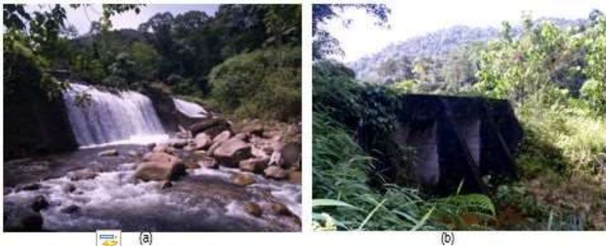
Fig. 1. (a) Mining dam which is located at the upper stream of Kampar river; (b) The pipeline supporting structure which are no longer in used and currently abandoned.
