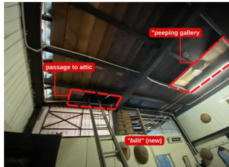
Figure 5 View of the 'passage to attic' and the void on the padong floor as seen from the tengah of House No. 1.
